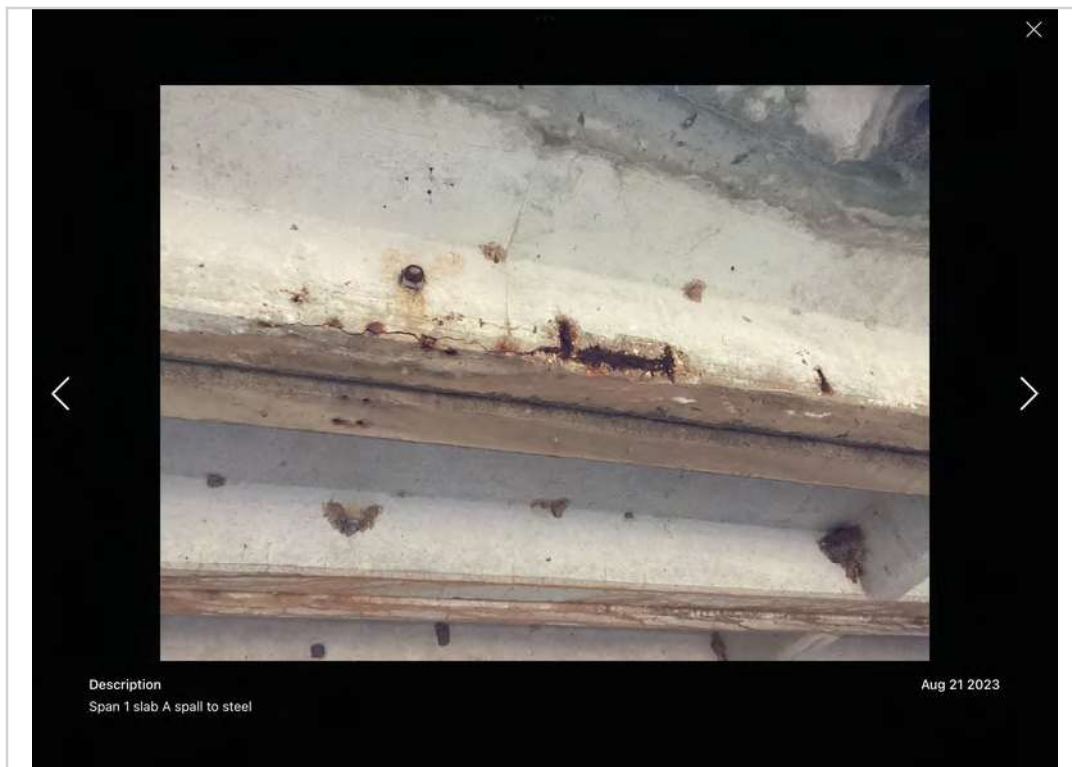
Span 1 slab A spall to steel
