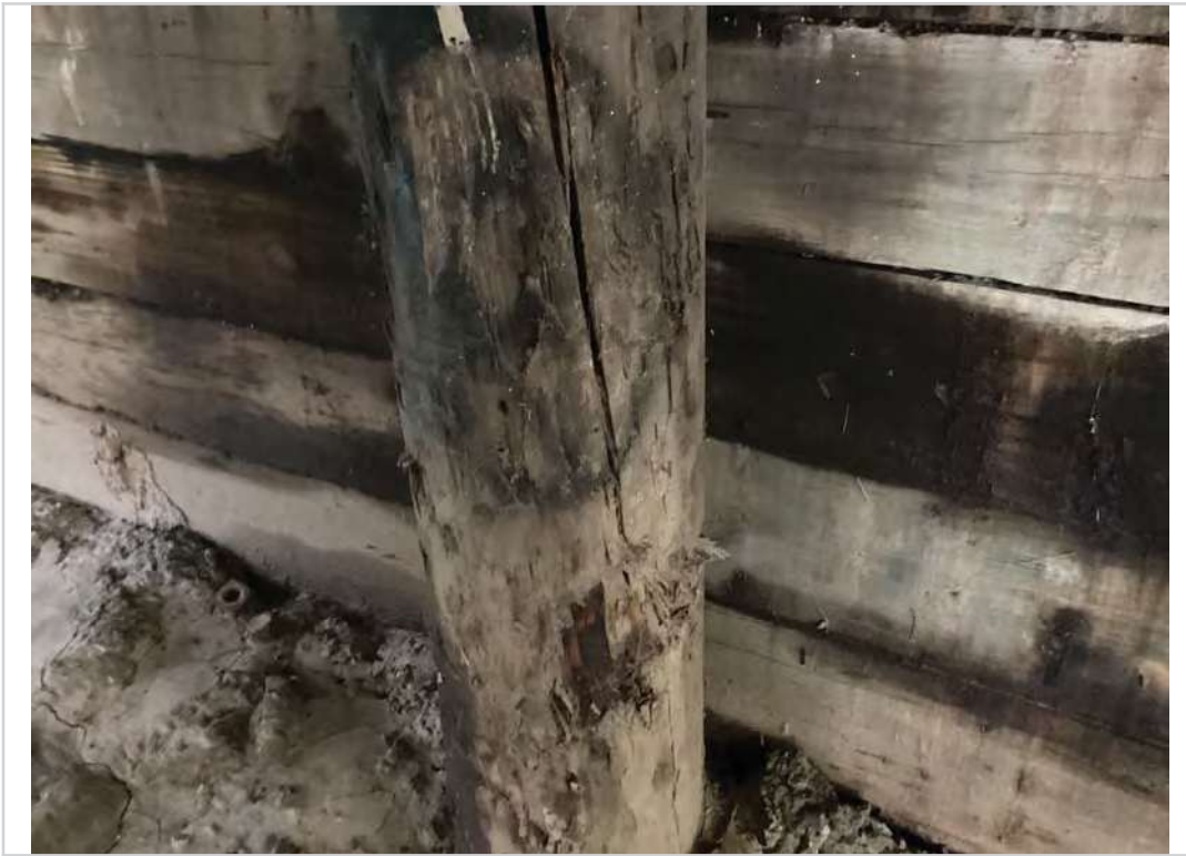
Split and splintering, pile C abutment 1
