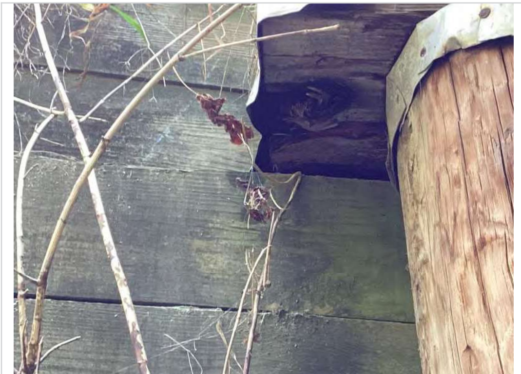
Abutment #2 cap splintering
