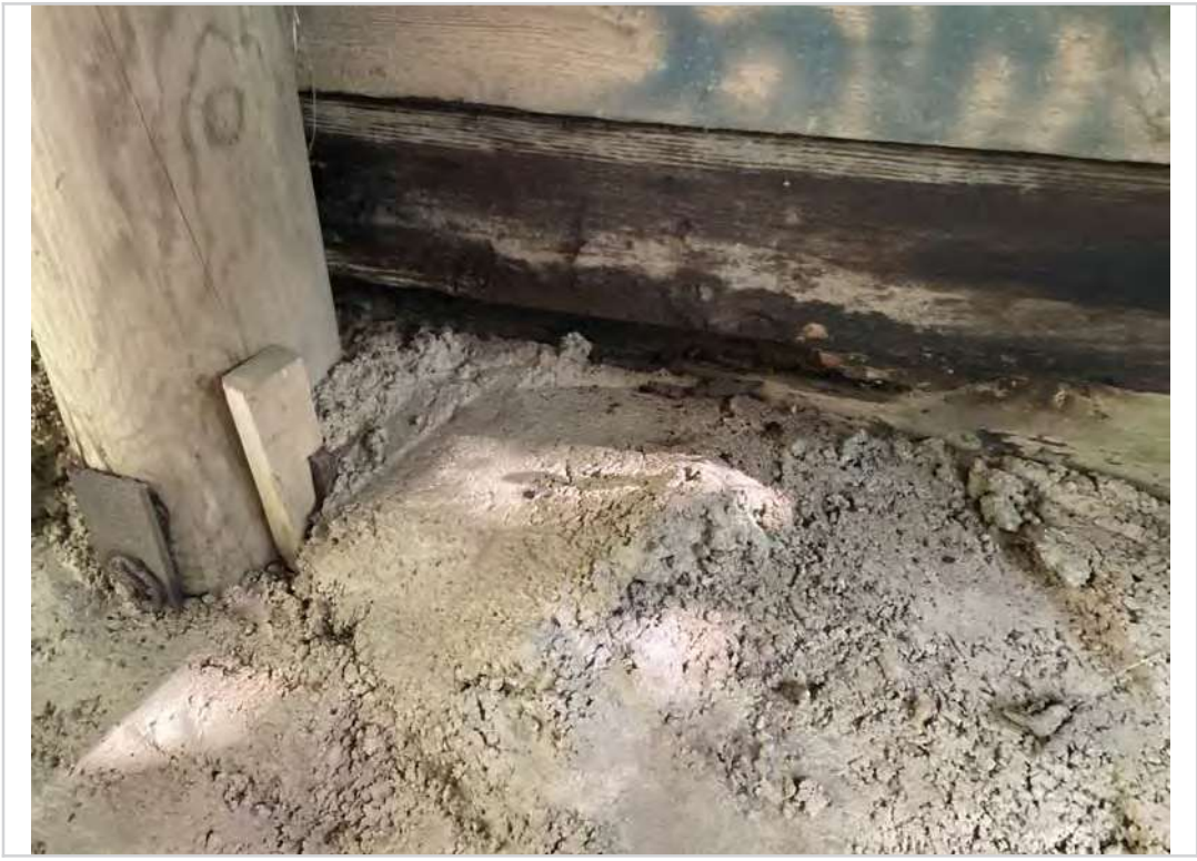
Abutment #2 breastwall decay
