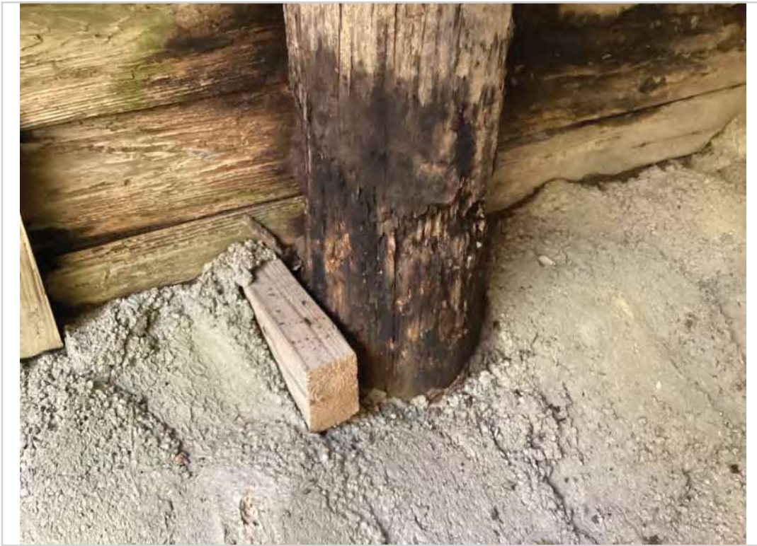
Abutment #2 pile B decay
