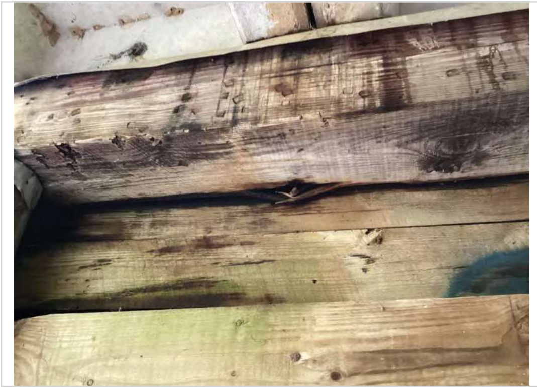
Abutment #2 cap splintering
