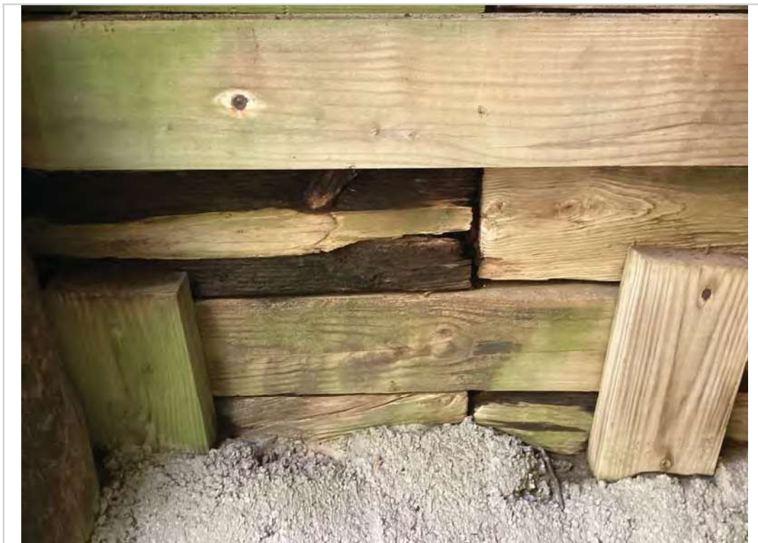
Abutment #2 breastwall decay
