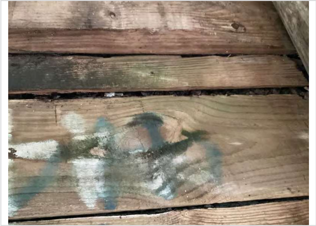
Abutment #2 breastwall decay
